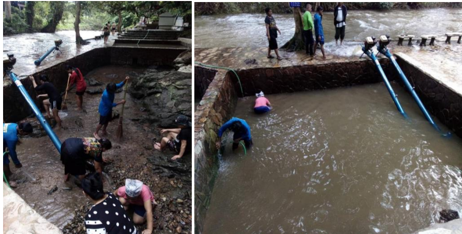
Figure 148: Cleaning Hin Dad hot spring after flooding (September, 2019)
