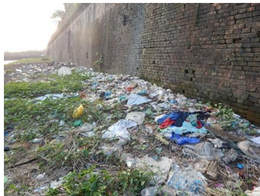
Figure 146. 3D Walls base, moats... easily become places of garbage stagnation
