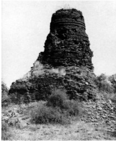
Figure 121: The Damaged Outer Stupa before Repair in 1997
