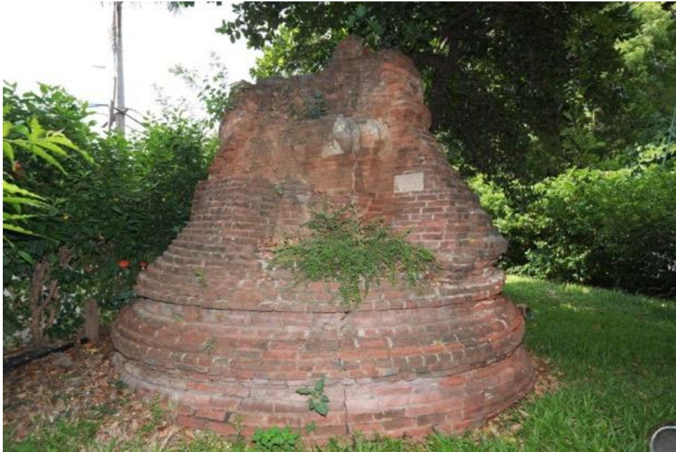
Figure 204: Monument No.1626 at the Old Bagan Area Note. Original inner stupa can be seen from the outside.
