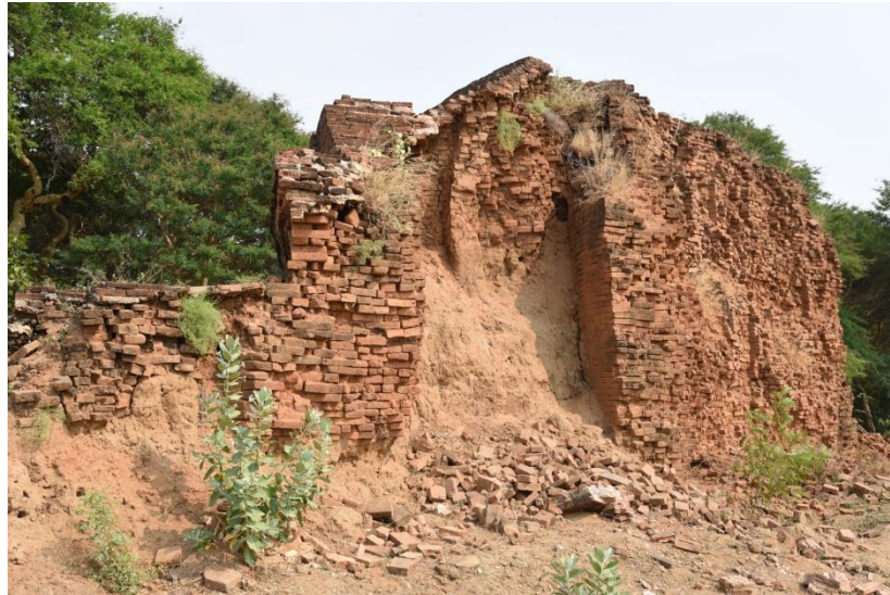
Figure 244: Part of inner stupa still remaining in this structure Note. There is a space with debris between inner and outer structures.
