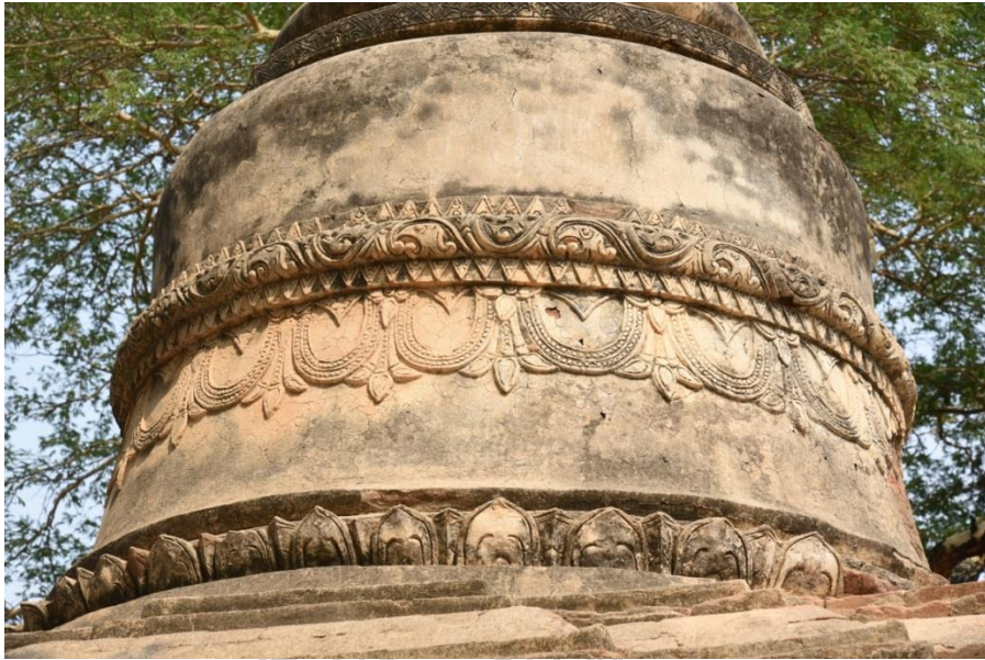
Figure 148: Original Stucco Decorations over the Bell-Shaped Dome Note. Original floral frieze around the waistband can be seen on the encased stupa.
