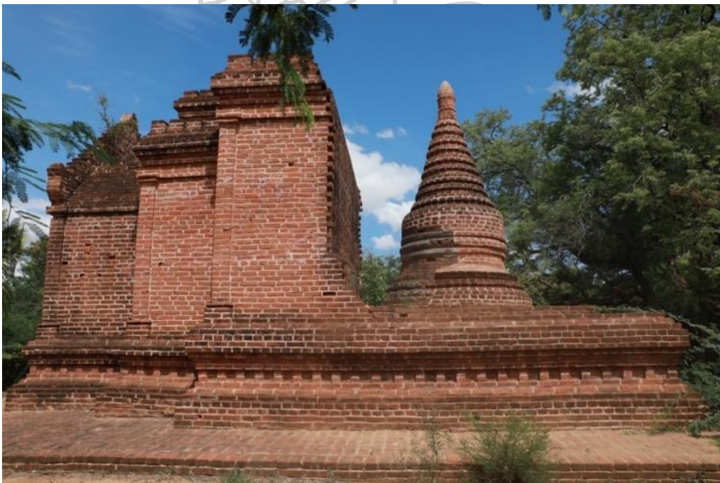
Figure 241: Monument No.1313 at the Myinkaba Area Note. The elevation of inner and outer monuments can be seen here.
