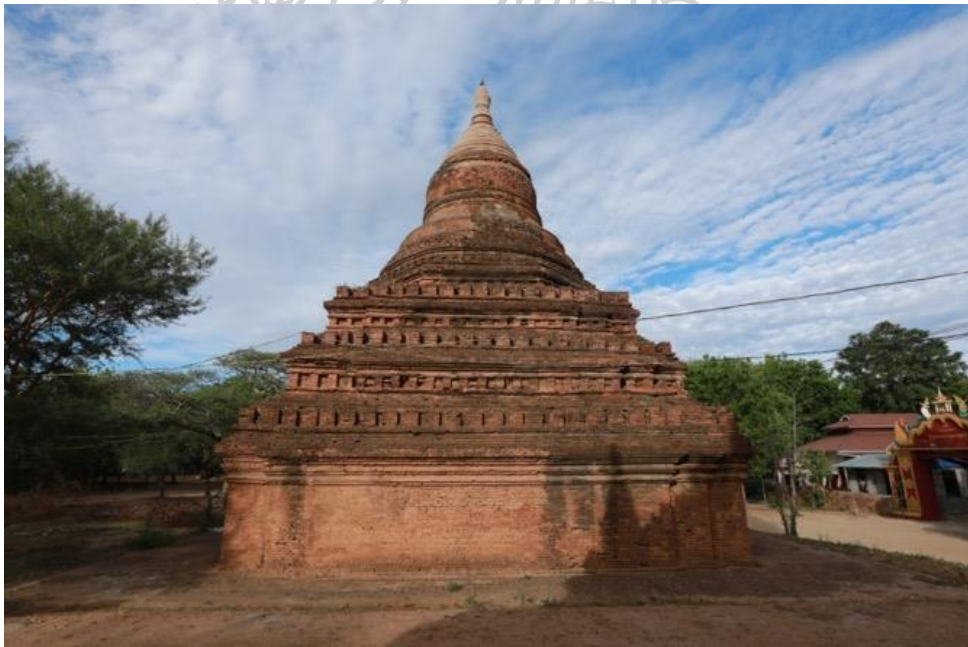
Figure 180: Monument No.1962 at the Taungbi Area Note. Inner stupa cannot be seen from the outside after repaired by the DOA.
