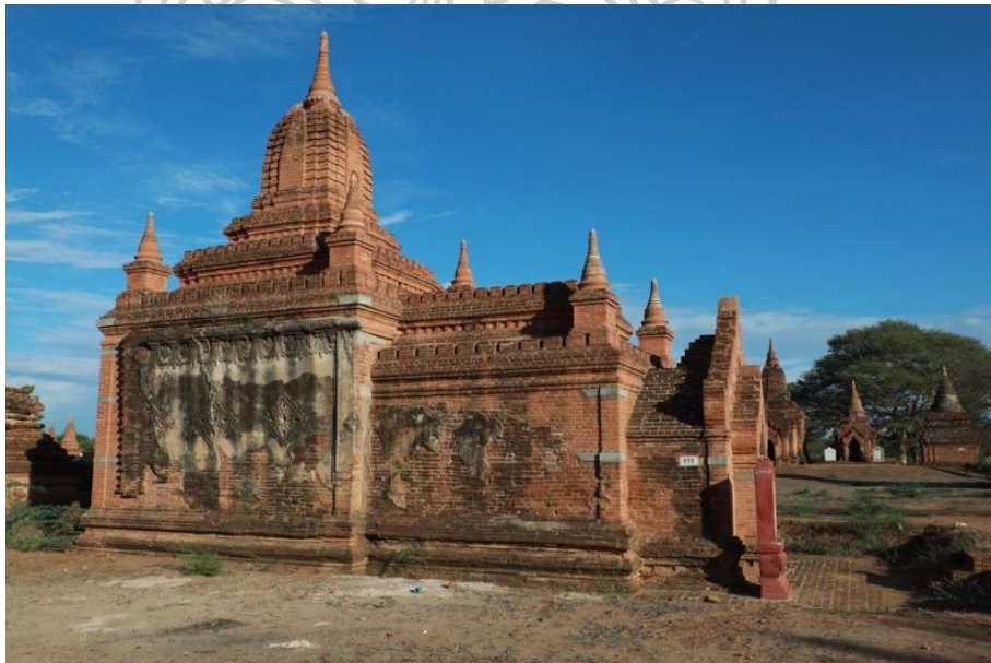
Figure 126: Monument No.347 (Wut-tha-na-daw Group) at the Wetkti-in Group Note. The false apertures in stucco on the north wall of inner temple can be seen here.
