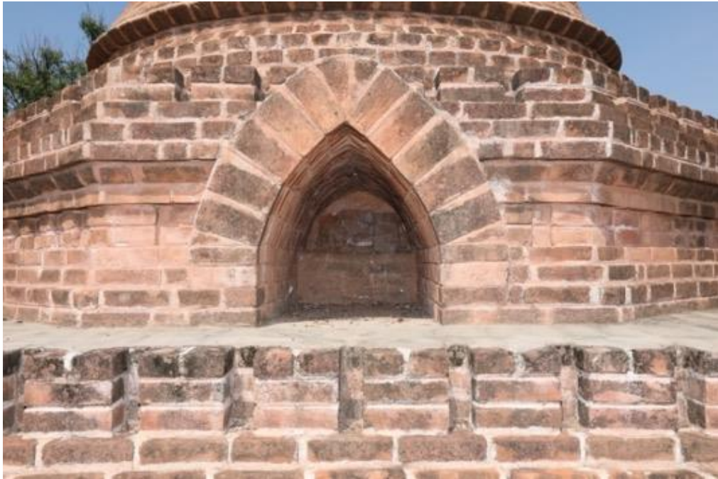
Figure 288: A niche with radiating arch exposed to see the encased stupa Note. Outer stupa was symmetrically built around the inner stupa.
