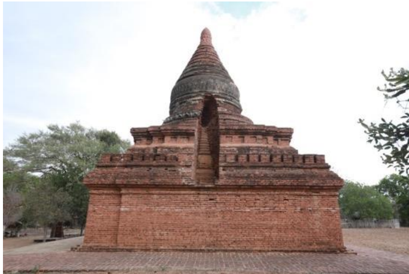
Figure 144 Monument of No.1689 at the Taungbi Area Note. The original inner stupa can be seen through a treasure hole from the outside.
