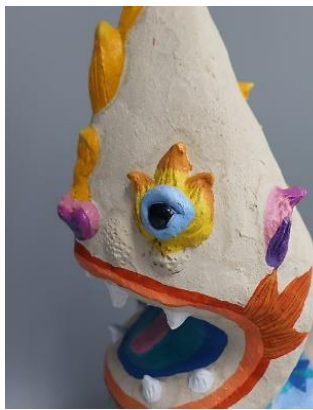
Figure 27. Tide lines staining from the second layer of stucco at the face area, Naga sculpture.
