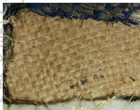
Fig. 84: Condition of the jacket in 2023, darkened area at the bast fibre lining.
