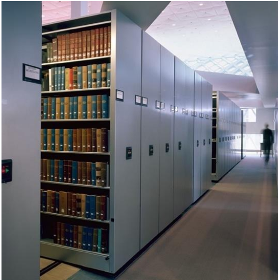
Fig 42. Electric Powered Mobile Shelving.
