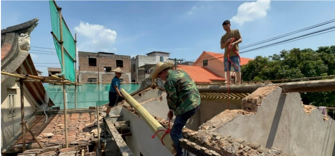
Figure 6: Southern Fujian buildings were damaged
