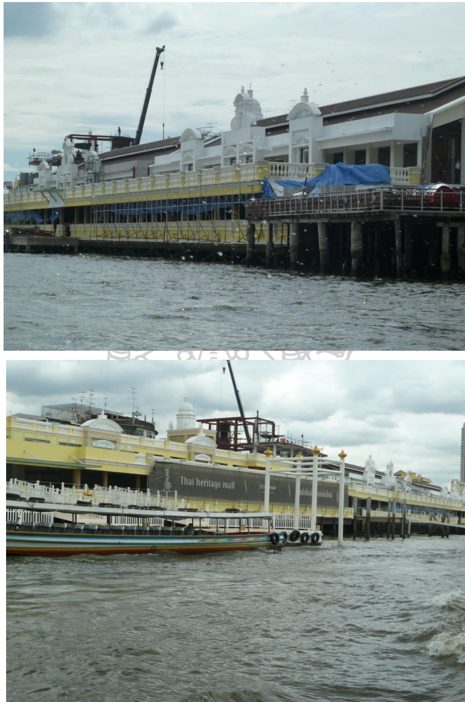
Figure 47A modern world of Rama VI: the new Pak Khlong Talat market under construction.
