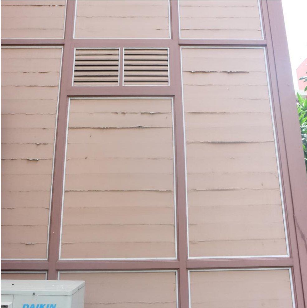
Figure 34 A section of a building exterior with rectangular panels in a pinkish-brown color. The panels are framed by brown borders. Some panels exhibit visible wear, such as peeling or cracking surfaces.
