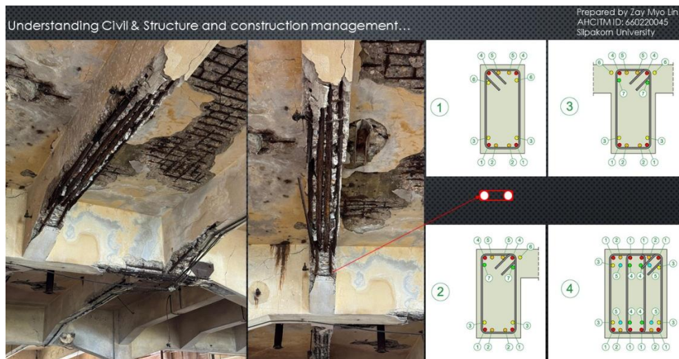
Figure 21: 4 type of beam founded as major group in Building B Photo and drawing by Zay Myo Lin, (2024)
