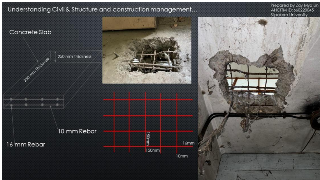
Figure 10: Building A, floor slab of level 1, ceiling of basement compartment Photo by Zay Myo Lin, (2024)
