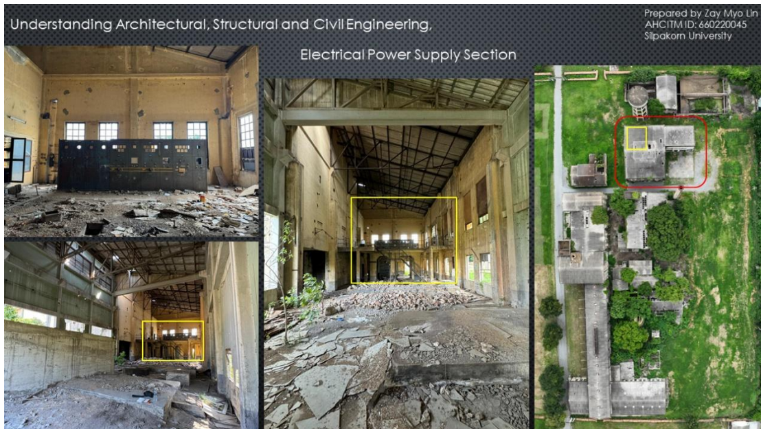
Figure 33: Electrical Power Distribution Sector at Building E Photo by Zay Myo Lin, (2024).
