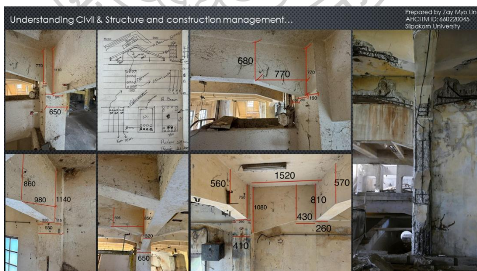
Figure 22: Stiffened concrete beam founded in Building B Photo and drawing by Zay Myo Lin, (2024)
