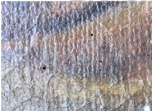
Figure 50: Small holes visible on the paint surface.
