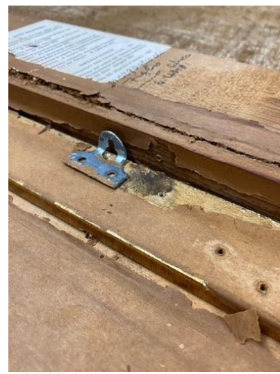
Figure 84: An L-shaped metal plate was removed from the original position.
