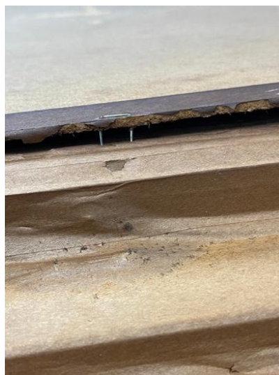
Figure 83: Doubled-legged metal staplers were tacked to the strainer.
